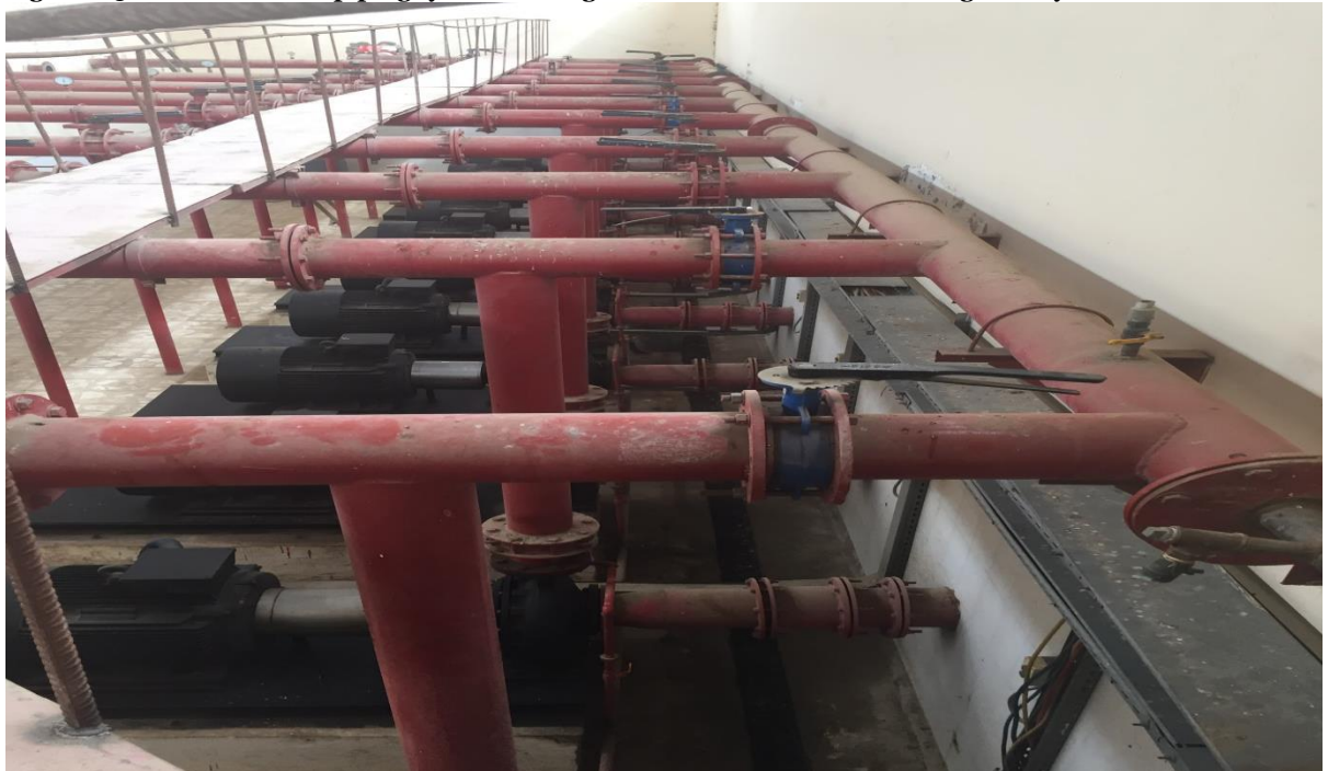
Figure 6.5. Industrial scale piping system feeding into the farms’ automated irrigation system
