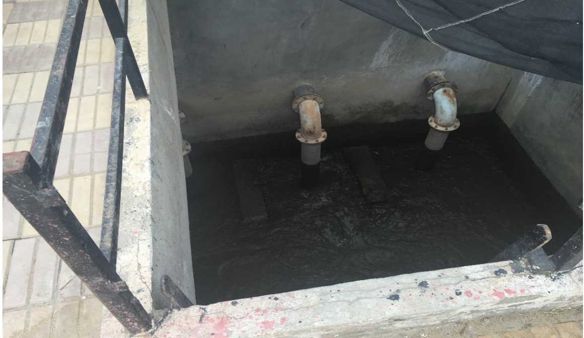
Figure 6.4 Pumps Intakes from tertiary canal feeding in the main station Salheya farmland
